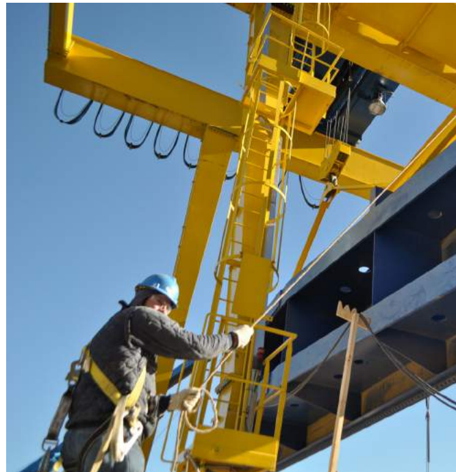
Angostura Power Plant
