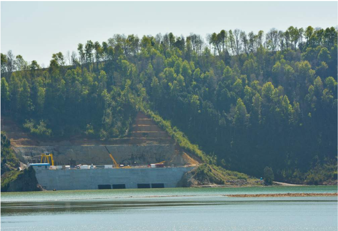
Angostura Power Plant
