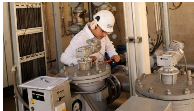
Hornitos Power Plant
