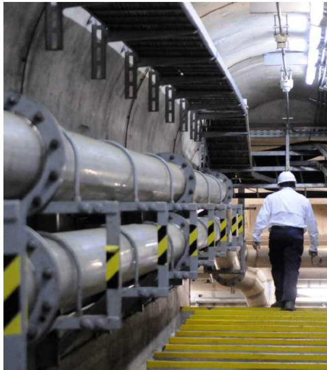
Power Station Colbún
