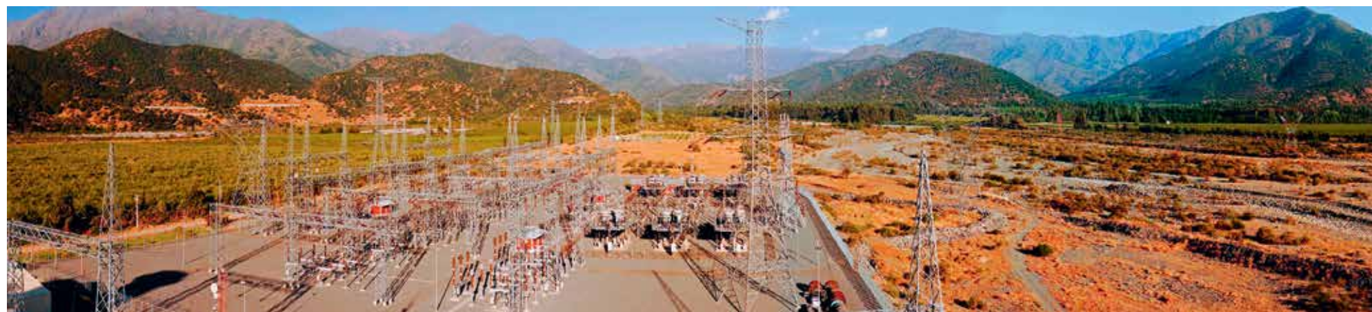
CANDELARIA POWER PLANT
