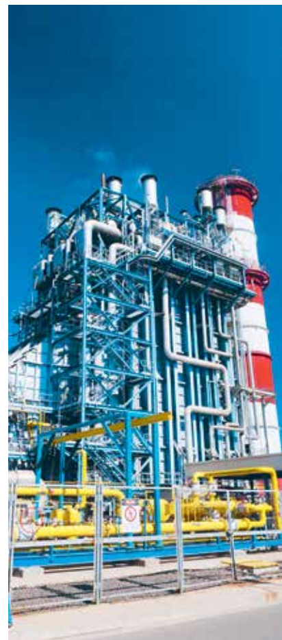
NEHUENCO POWER PLANT
