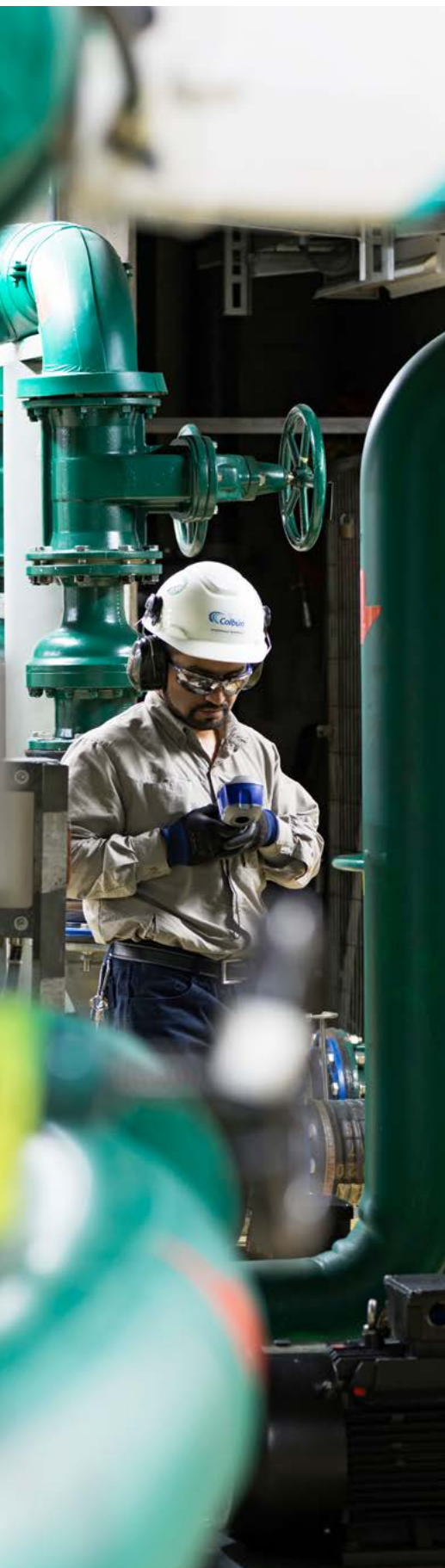
Cavern Canutillar Power Plant, in Los Lagos Region
