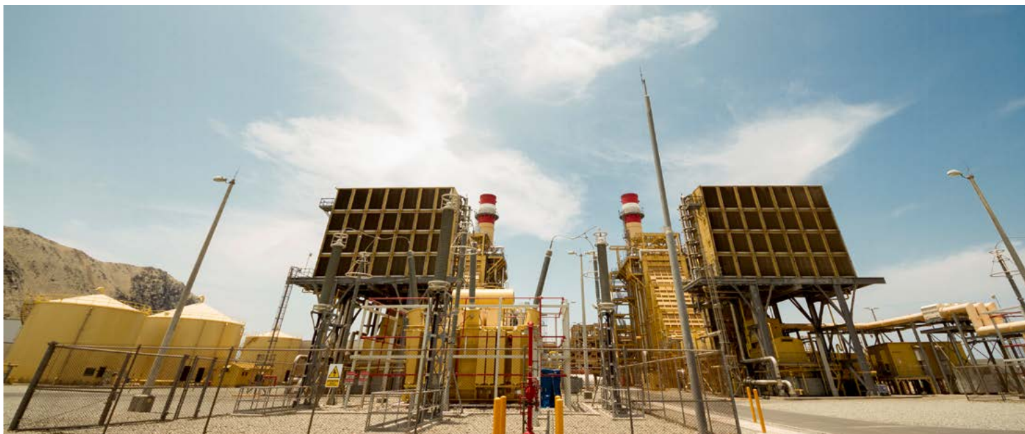
The two units of Fenix Power Plant, Chilca, Peru
