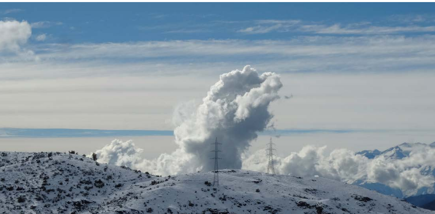
Transmission towers in the Aconcagua Valley. Picture by Jorge Jaramillo, Aconcagua Complex
